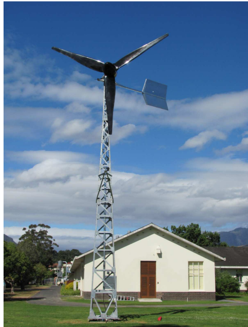
Figure 3: Antarctic 20 kW wind generator
