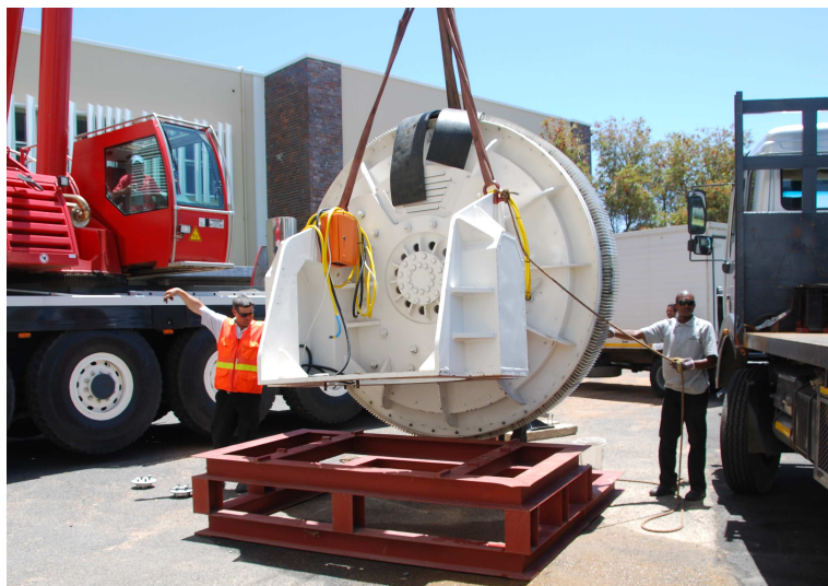
Figure 4: Unloading the 300 kW permanent magnet generator for testing at the EMLab.
